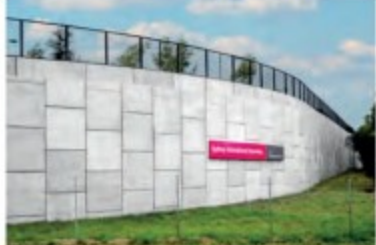
Top: The new speedway comprises several precast elements, contributing to a world-class facility.
