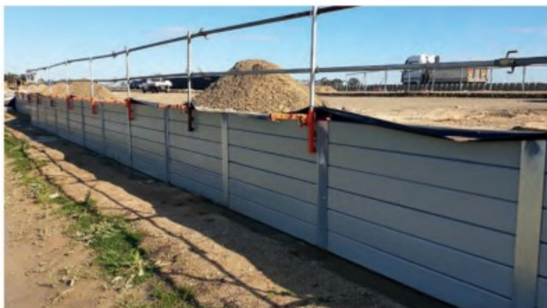
PROJECT: Koo Wee Rup Bypass CLIENT: VicRoads HEAD CONTRACTOR: Lend Lease Engineering PRECASTER: Sunset Sleepers
