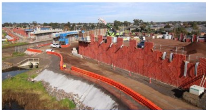
PROJECT: Barwon Heads Road Upgrade LOCATION: Barwon Heads, VIC MASTER PRECASTER: The Reinforced Earth Company Australia
