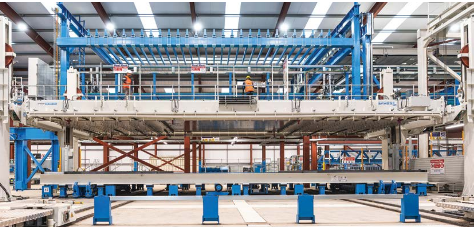
ABOVE: Installed by Ebawe Anlagentechnik, the state-of-the-art turning equipment delivers an almost flawless surface quality.
