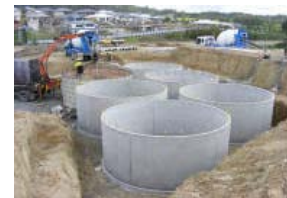
Man falls 6m into concrete tank (QLD)
