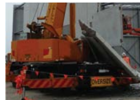
Alert: Precast erection failure (VIC)
