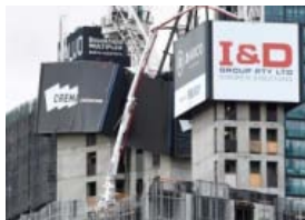
Collapsed crane causes chaos (VIC)
